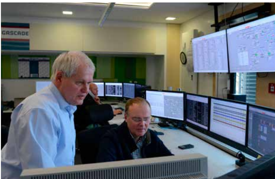
Dispatching centre at GASCADE.
