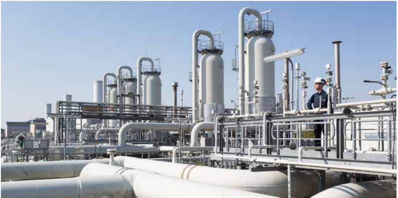
The GASCADE pipeline network is a hub for European natural gas transport.
