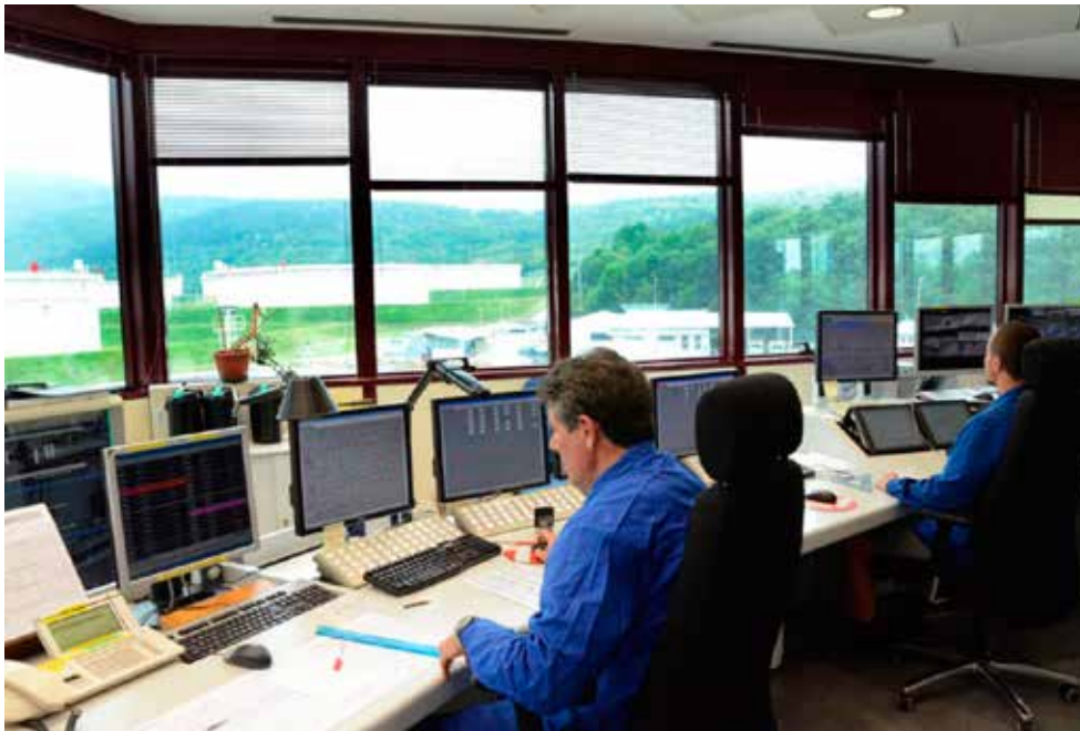
Monitoring and control of the pipelines and plants at TAL.
